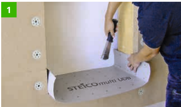
Attachment of STEICOmulti UDB (diffusion-open membrane) as temporary weather protection until window installation.
