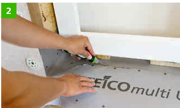
The windows are installed on the membrane. Before STEICOfix is installed, the sheet is cut back „half-moon-shaped“ (see Fig. 5).
